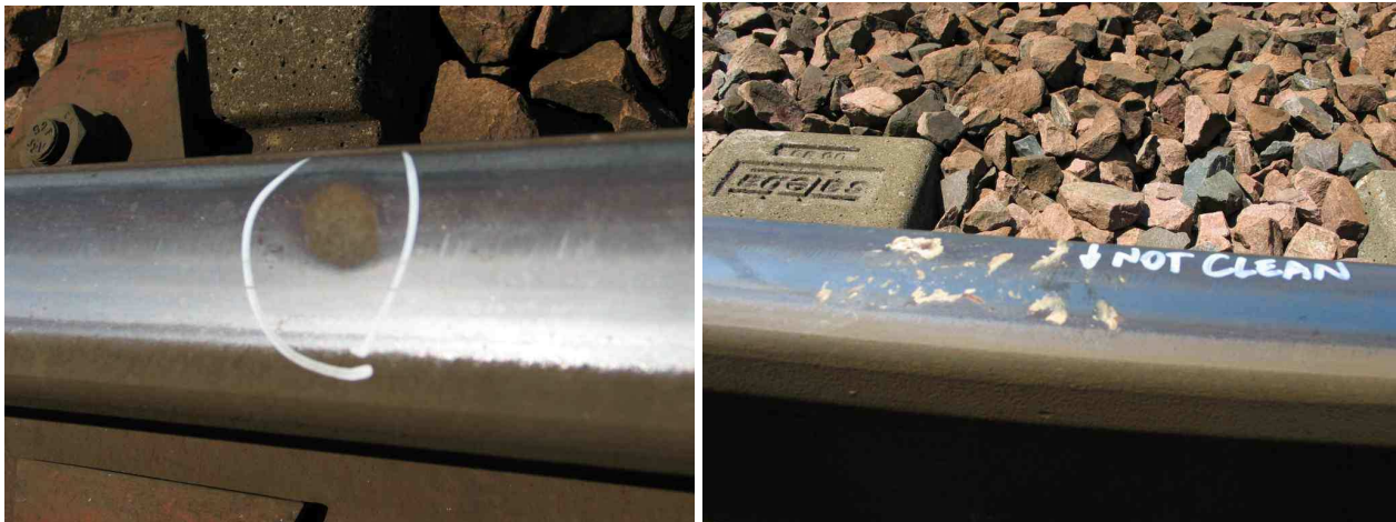
Figure 5. Ballast print (left) and dried bird droppings (right): typical defects of outside track in country areas.
