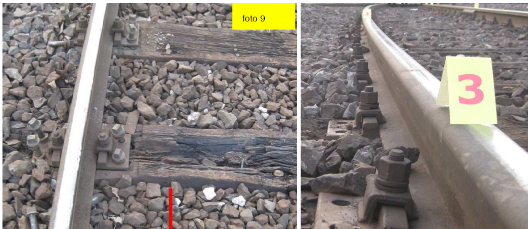
Figure 4: Aged conditions of wooden sleepers on the turnout in Chiasso responsible for the derailment of a locomotive.
