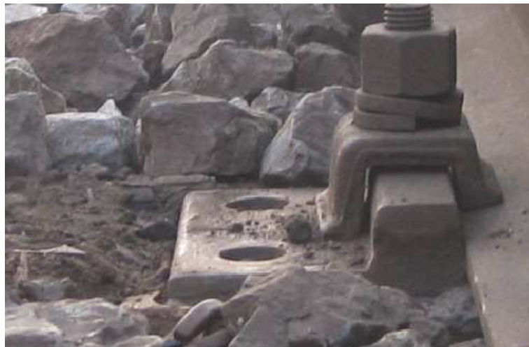
Figure 5: Detail of the baseplate with missing coach screws.
