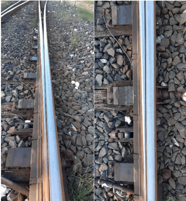
Fig. 4. Above: an expansion joint (source: Internet). Below: Switch rail/stock rail pair of a heavily loaded turnout (Photo A. Bracciali, Florence, July 09, 2022).
